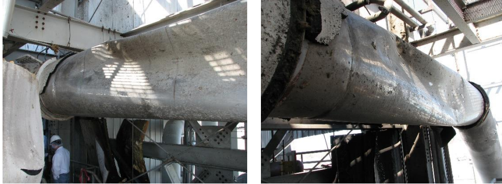
Figure 10. A duct (featured from two angles) that collapsed.
