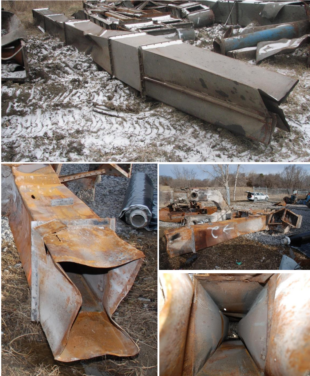
Figure 11. Collapsed rectangular duct. Note that the shorter section in the top photograph did not collapse, whereas longer sections did.
