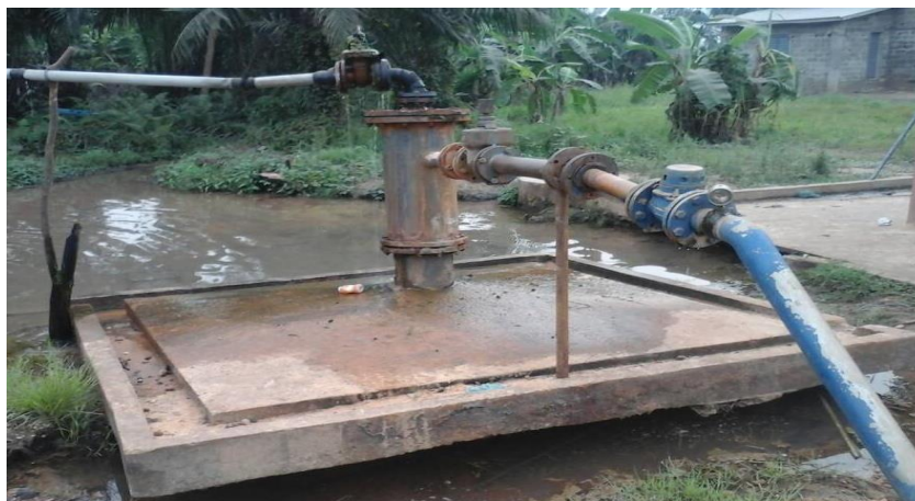
Figure 5. Damaged wellhead equipment [2]
