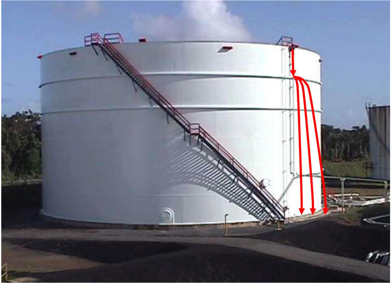
Figure 4 Fixed Roof Tank Showing Stiffening Rings and Spill Trajectory Into a Spray Cascade
