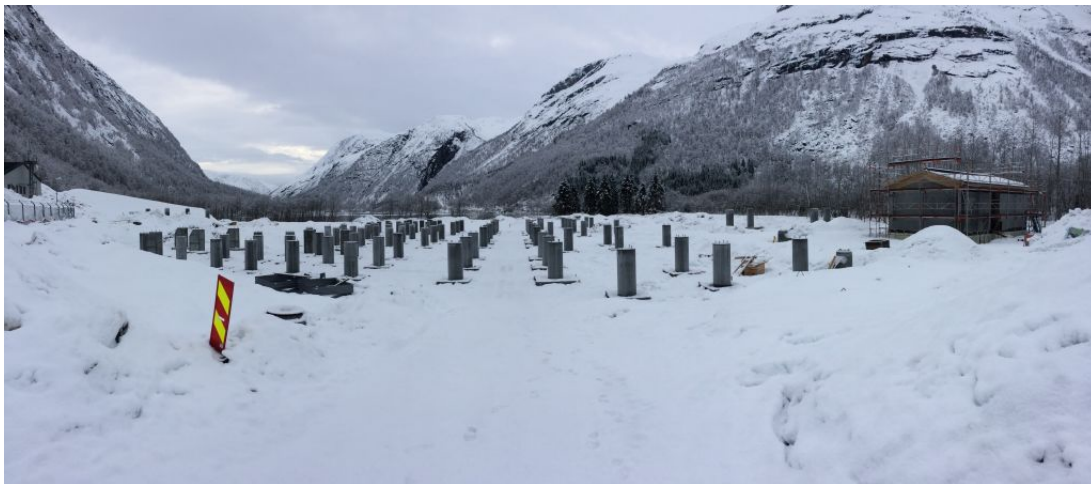
Figure 1.2: 300/420 kV outdoor switchyard under construction. Shows a facility of 3200 m 2 with concrete pillars of approx 2-2.5 m heights for equipment. Grounding grid to be buried in soil at 0.6 m depth from top of the pillars to give equipment grounding connection
