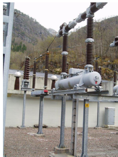
Figure 1.3: Typical infeed arrangement in an outdoor switchyard for a domestic hydropower station
