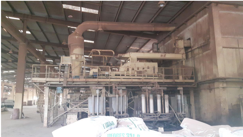
Fig. 4. Chemical/blending working section (Photo: Akeza)
