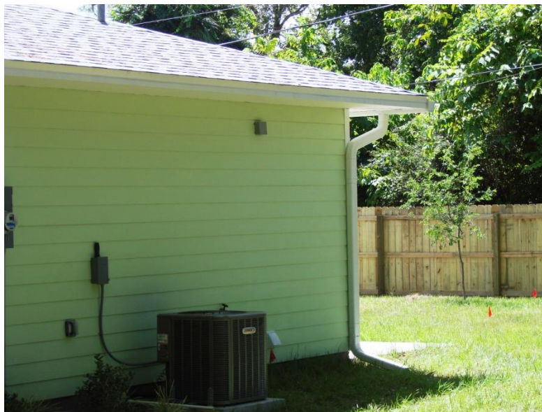
Figure 7. SEVHFH ran conduit from the electrical panel to a junction box (Seen high on the wall) to facilitate future installation of a solar electric system.
