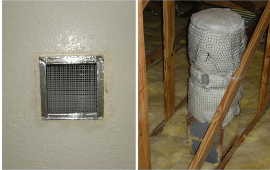
Figure 2. Ceiling penetration for planned leakage (left); attic view of hole that diffuses airflow (right)
