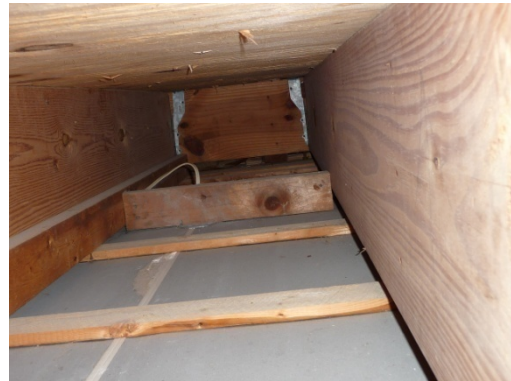
Figure 88 View from inside west soffit, evidence of complimentary air pathway at back of photo.
