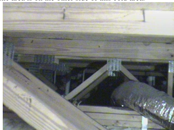
Figure E-6 Photo of image at left. View is facing east into 14" high 2 nd story floor space in the main part of the house.
