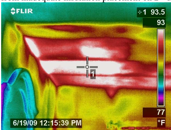
Figure 163 Area of front left 2 nd fl. bedroom with very hot ceiling due to inadequate insulation placement.
