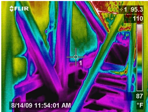
Figure E-13 IR view inside the hot attic shows cooled surfaces low in attic in H16B before repair.
