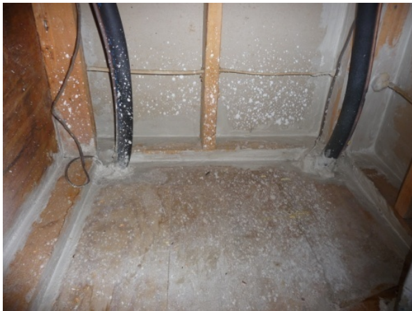
Figure 77 1 st floor system return plenum with effective air barrier at all joints and penetrations.
