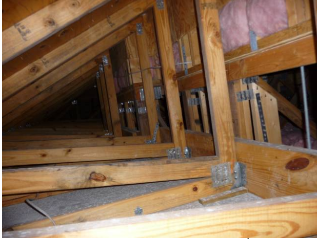
Figure 169 North attic section with open 2 nd story floor space. Insulation batts are located inside the floor space on the ceiling of the first floor.
