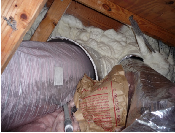
Figure 103 East side floor cavity isolated from the garage attic; a protective vapor barrier/thermal barrier sleeve isolates the foam from the exterior of the supply ducts.
