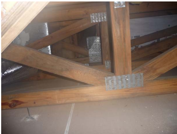
Figure 136 Open floor cavity area in the east attic. (view looking toward the west into the floor space)
