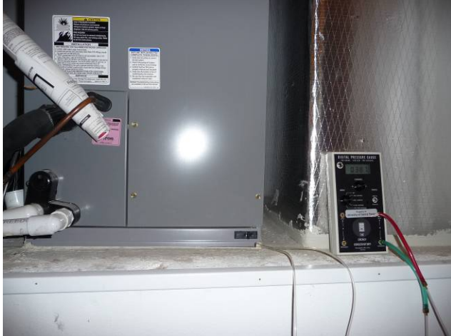
Figure 176 Air handler in garage has typical panel leakage at seams and penetrations.
