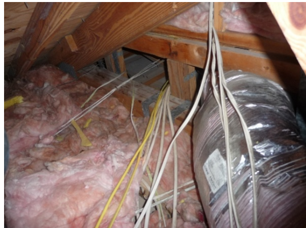
Figure 98 Supply duct running into an open floor cavity in garage attic kneewall.
