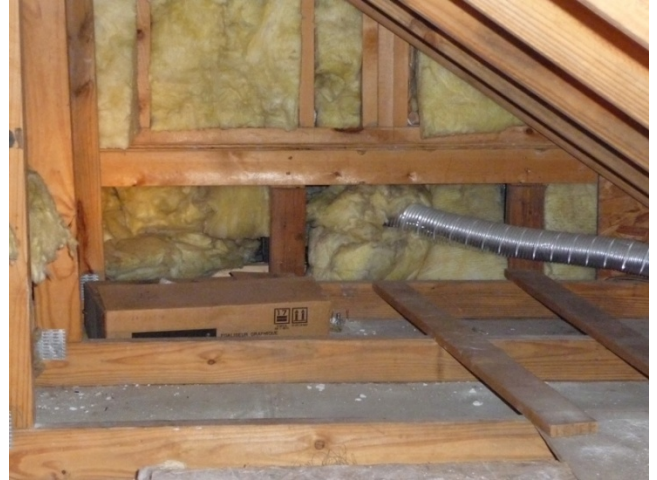
Figure 28 Kneewall partially blocked adjacent to floor space
