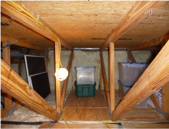
Figure 48 H7 inside bonus room floor space facing south. Batts separate floor space from a small vented attic area.
