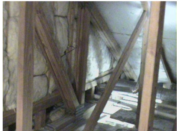
Figure E-14 Photo of IR image to the left. The floor cavity at the bottom of the wall is open to attic space.
