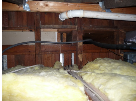
Figure 74 Floor cavity directly connected to attic area.
