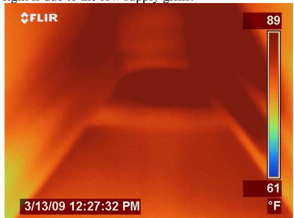
Figure 34 IR image showing very hot areas of ceiling and air infiltrating from the garage attic.
