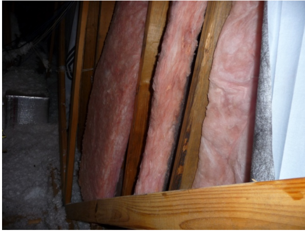
Figure 159 Stairway kneewall view from attic with batts away from wall.
