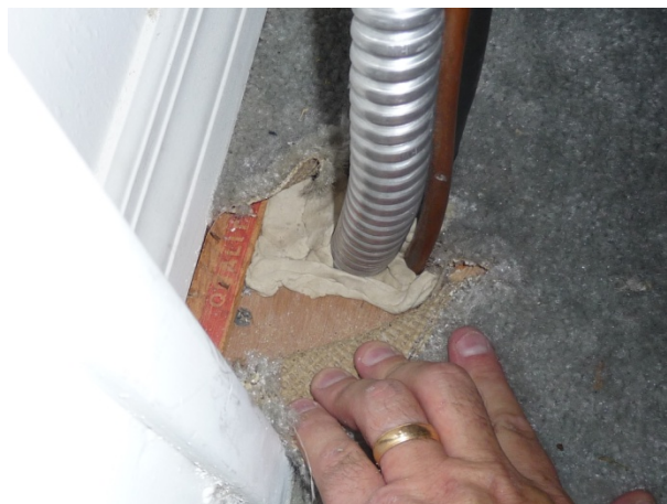
Figure 80 Conduit and refrigerant line penetrations were sealed on the second floor system.
