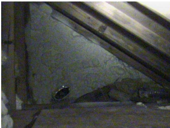
Figure 39 Kneewall on opposite side sealed with foam.
