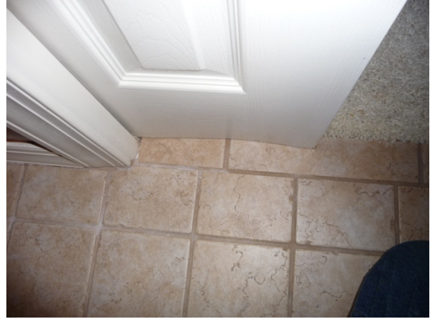
Figure 84 Warped pocket door from air infiltration from north attic area.
