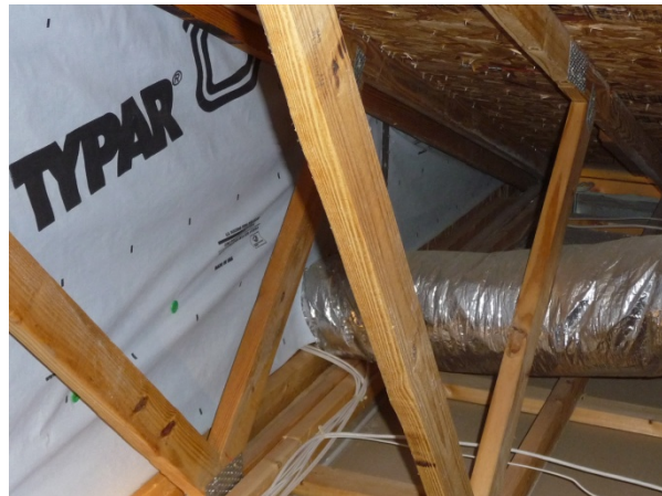
Figure 158 Portions of kneewall and floor space were covered with plywood and house wrap.
