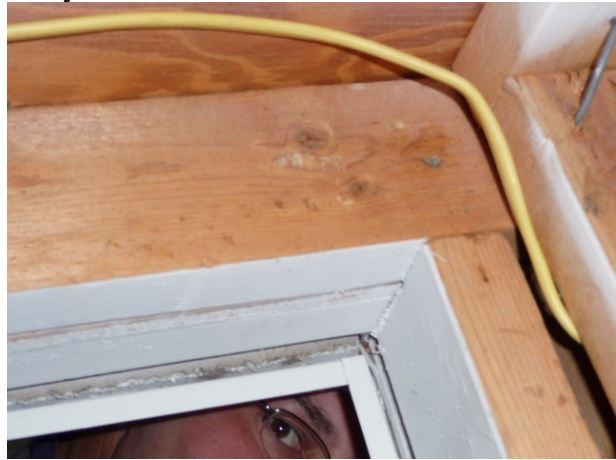
Figure 76 A view from inside the return plenum shows a lack of sealant or air barrier in return plenum.
