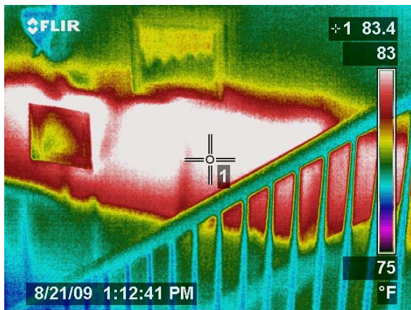
Figure 19 Infrared image of floor space behind wall.
