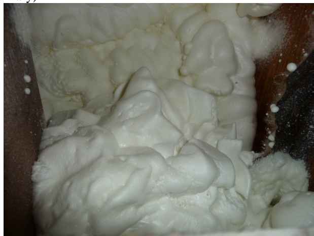
Figure 126 South side insulation applied over top of floor deck, then floor space vertically sealed off by foam wall from floor deck down to bottom of floor space.
