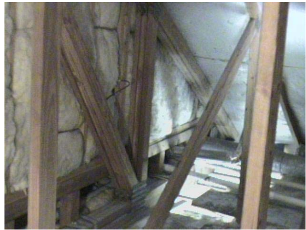
Figure 107 Photographic view of IR image to the left. The interstitial floor cavity at the bottom of the wall is open to garage attic space.
