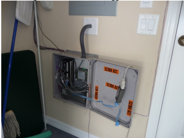
Figure 23 Datalogger seen inside enclosure with door open and located below electric service panel.
