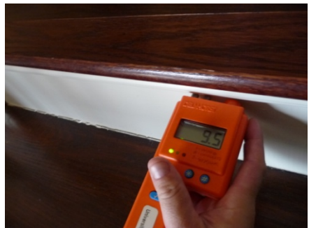
Figure 93 Moisture content readings were about 13% at top of stairs with trend that fell to about 9.5% at bottom of stairs.
