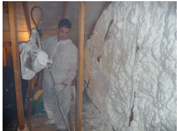
Figure E-12 Insulation tech just finishing up kneewall and floor insulation/ air tightening (H16B).
