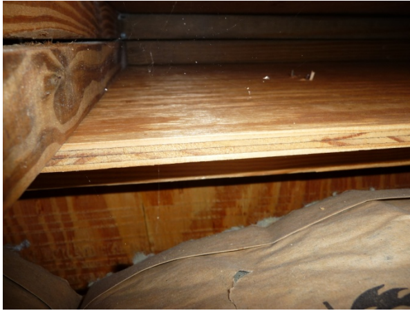
Figure 1446 View looking up into open wall cavity from east attic shows no insulation in this wall next to walk-in closet.
