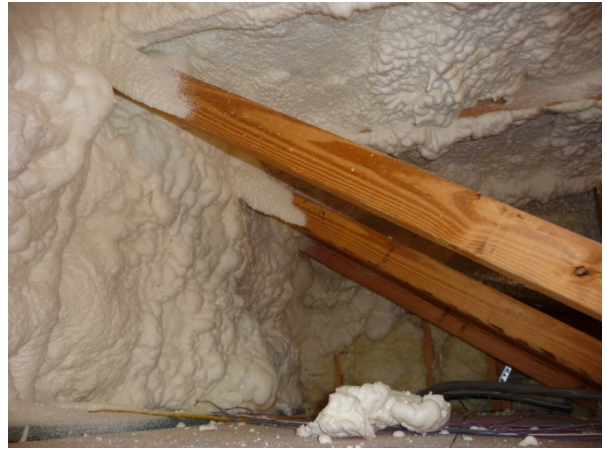
Figure E-8 Foam applied to wall and ceiling of the bonus room (3' high) floor cavity.
