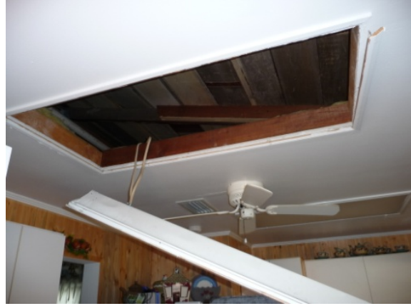
Figure 72 Access to attic space through light fixture opening in kitchen ceiling.
