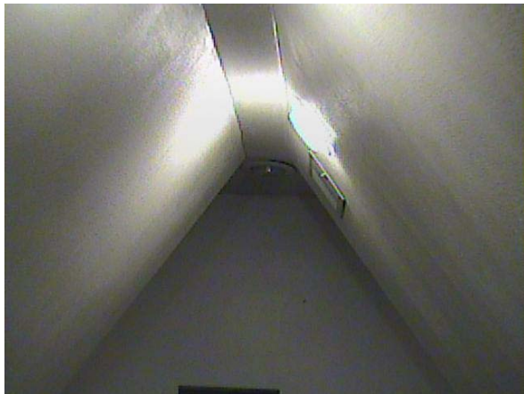
Figure 33 Ceiling of bonus room with leaky recessed light.
