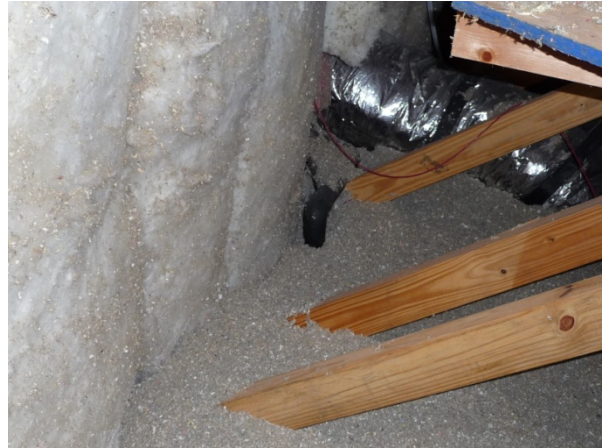
Figure 14 In House H22, batts and blown insulation cover the opening to floor cavity.
