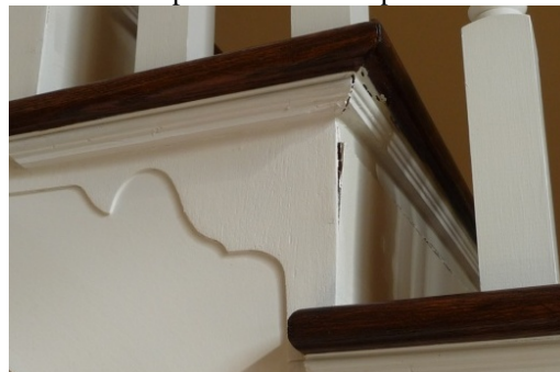
Figure 94 Cracking and separation before repair.
