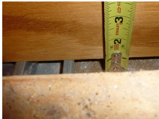
Figure 4 Photo from inside attic at House H13. A 1” gap exists between plywood that covers the kneewall and the 1 st floor ceiling below. This gap allows air to flow from the attic space to the 2 nd story floor cavity.
