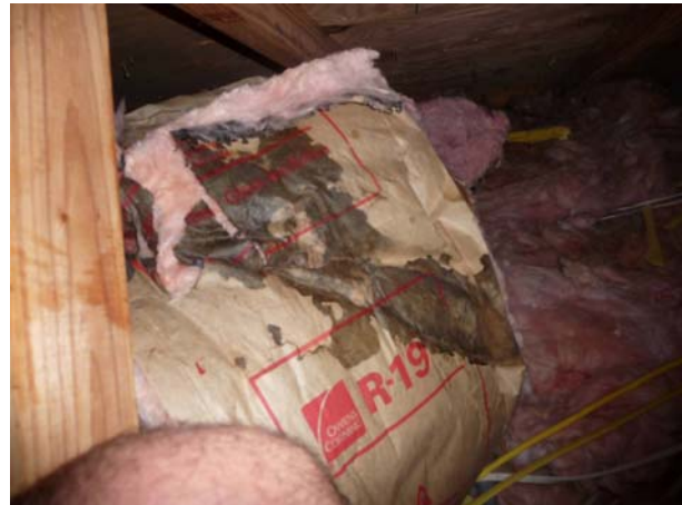
Figure 130 Batt pulled away from duct shows it is soaked where dark areas are seen on paper facing.
