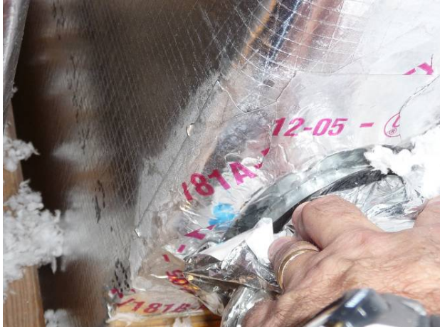
Figure 174 Flex duct connection with no mastic on first floor return plenum. Flexduct is mechanically fastened, but not airtight.
