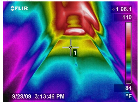
Figure 42 heat transfer through the bonus room walls is high in upper sections which are close to attic roof deck.
