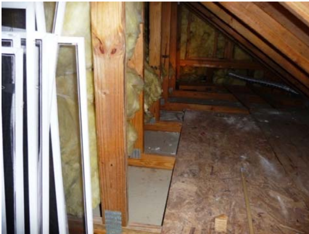
Figure 29 View of kneewall, floor space (far), and bonus room wall. Unsealed floor cavity is to the left.
