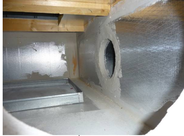
Figure 175 Inside of 2 nd story support platform sealed well with mastic on seams and duct connections.
