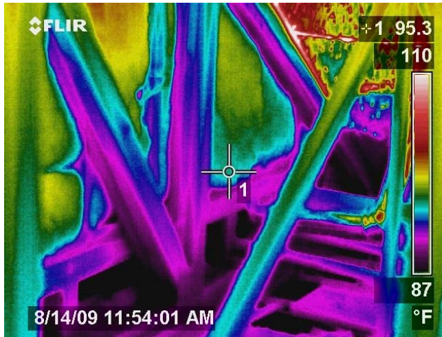
Figure 106 IR view inside the attic shows cool temperatures in the floor space and cooled surfaces low in attic.
