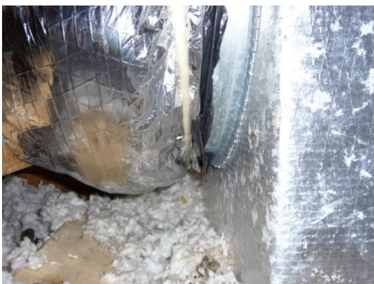
Figure 5 In House H2, a loose fitting flex duct creates part of a large return leak.
