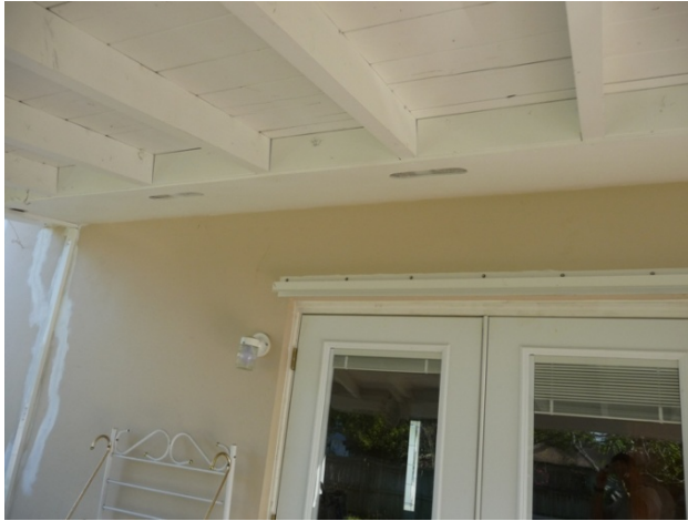
Figure 116 Cantilevered section of floor space on south side showing 2 of nine vent openings.
