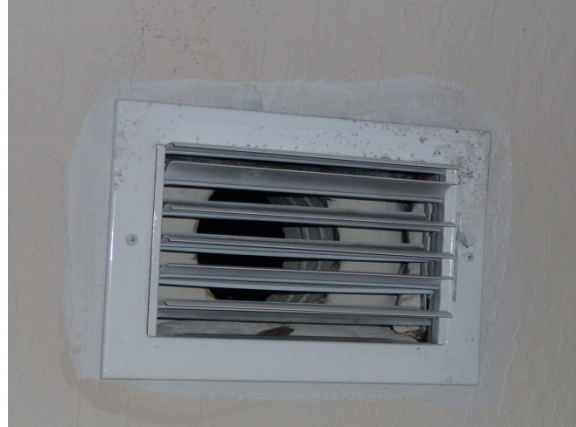
Figure 96 Evidence of condensation damage, mold and recent repairs by homeowner.
