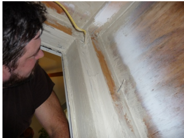
Figure 78 Mastic properly applied reduced return leaks from unconditioned space.
