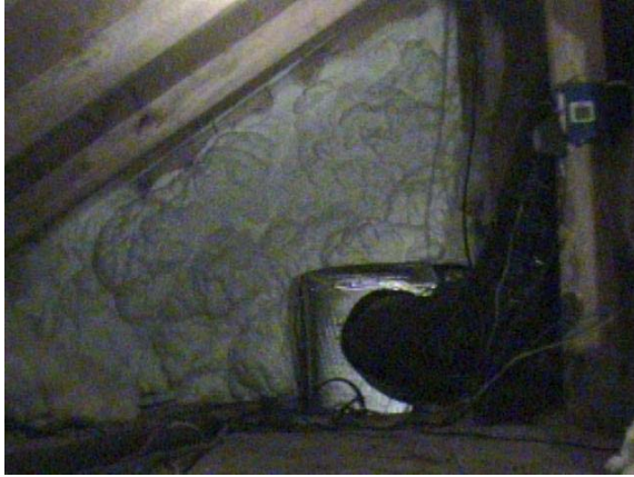
Figure 37 Kneewall effectively sealed with foam product. Duct penetrations were wrapped with a foil faced insulation product to prevent moisture condensation.
