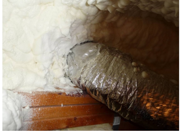
Figure 132 Supply duct from attic to floor space with insulation wrap around duct after foam applied.
