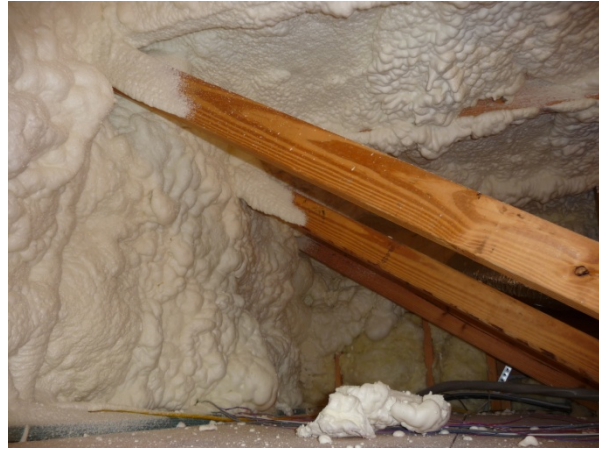
Figure 65 Foam applied to wall and ceiling of the bonus room (3' high) floor cavity.
