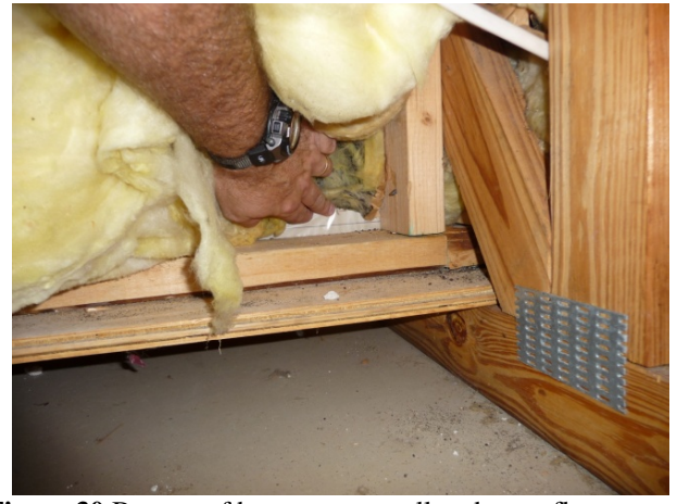
Figure 30 Bottom of bonus room wall and open floor space as seen from garage attic. Wall assembly (as described above) is also evident in this picture.
