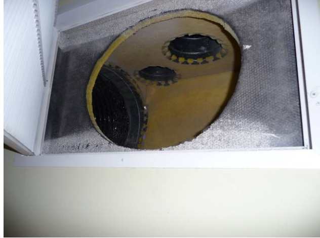
Figure 173 Main return for first floor with undersized opening into return junction. View inside box shows return ducts (from left to right) 20" diam. flex to main plenum, office, and master bedroom.
