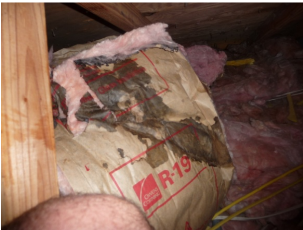
Figure 97 Moisture damaged batt.
