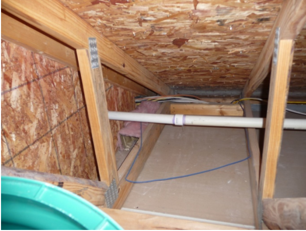
Figure 12 No wind washing potential was found in House H18 because the kneewall insulation and floor cavity are covered by plywood.
