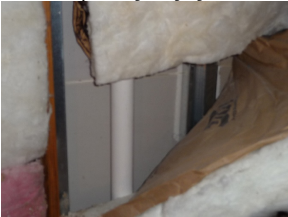
Figure 15 In House H22, an area of fallen batt on kneewall allows hot attic air to transfer heat through wallboard into conditioned space.
