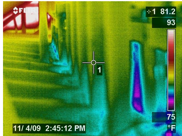
Figure 172 IR image of open floor space with east hip roof section in background shows roof deck only 93 deg. F. North attic section about 89 deg. °F.
