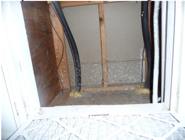
Figure 75 Leaky return plenum.
