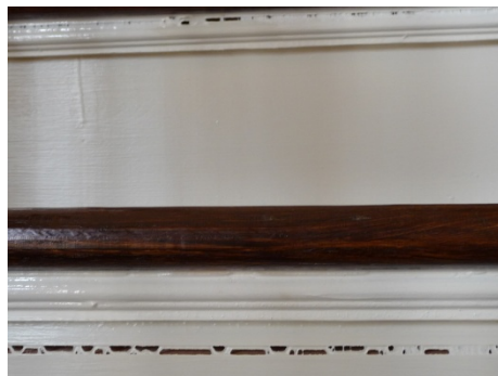
Figure 92 Riser separation before repair.
