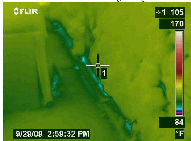
Figure 113 IR image from inside attic after repair.
