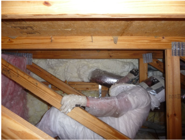
Figure E-7 Technician applying foam to opening between the 2 nd story floor cavity and the bonus room floor cavity (H7G).
