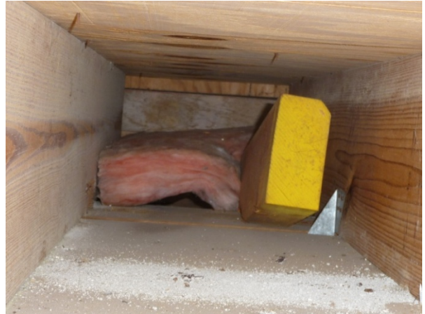
Figure 116 Kraft faced batts located inside cantilevered portion of floor deck in most bays. Most only partially block opening from vent space to floor area. View from inside looking out to patio south side.)
