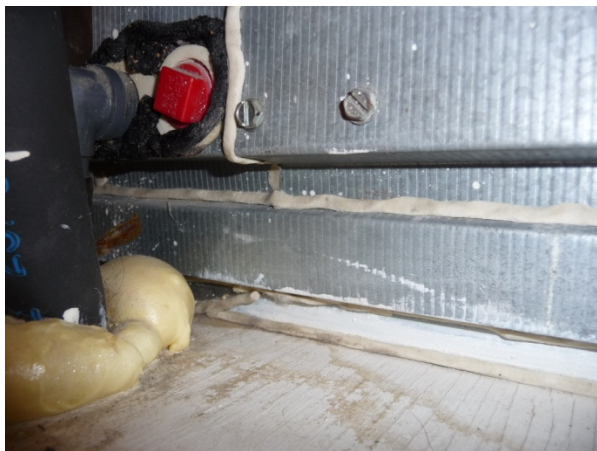
Figure 79 AHU leaks sealed with expanding foam and caulk on first floor system.
