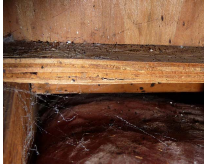
Figure 120 View of air leakage between batt and floor deck on north side facing South. Air leakage estimated to be about 2"x 22" in each bay.
