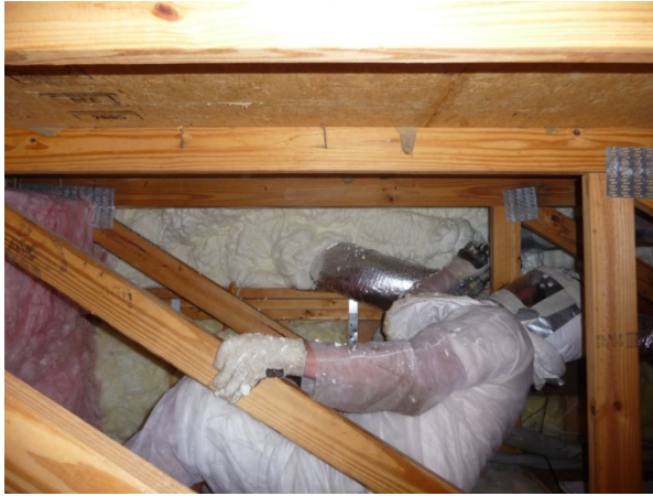
Figure 64 Technician applying foam to opening between the 2 nd story floor cavity and the bonus room floor cavity.
