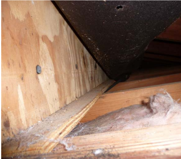
Figure 119 North attic section looking west from garage attic. North soffit vents are to the right. Felt paper being held up to view small kneewall area not insulated and floor space at bottom.
