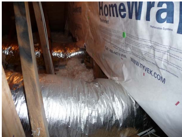
Figure 137 Open floor cavity area in the west attic. (west side is to the left)
