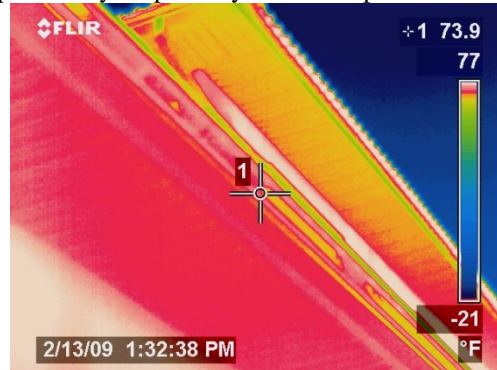
Figure 90 IR North soffit.
