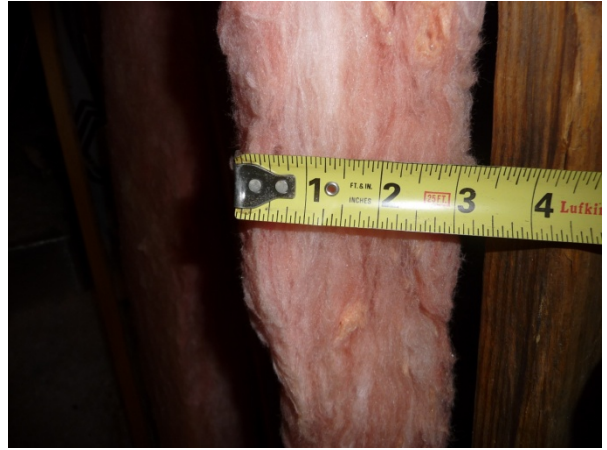
Figure 160 Air space between R11 batts and wall allow hot air in contact with interior drywall.
