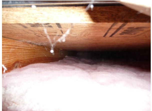
Figure 16 A view inside the floor cavity of House H22 shows that batt insulation is lying on top of 1 st floor ceiling, providing a thermal barrier to heat flow through the ceiling, but not through the floor of the 2 nd story. These batts were used only where garage portions were below 2 nd story conditioned space.
