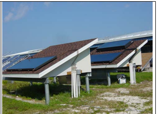
Figure 1- 28 The solar collectors, with the ICS system in the rear top
