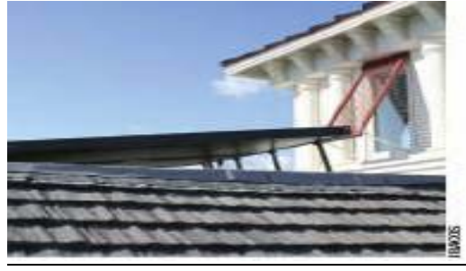
Figure 2- 34 Solar water heater on TNAH 2008
