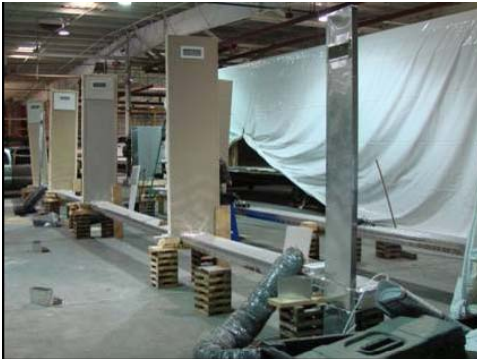
Figure 1- 2 Floor duct system with high side discharge outlets under construction being tested with duct tester.
