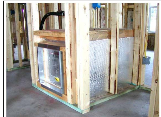
Figure 4- 15 Detail of a ducted return air plenum
