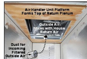
Return plenum with ventilation duct. ~25cfm of outside air enters return plenum when air handler is operating
