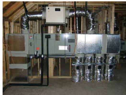
HVAC Equipment Installed
