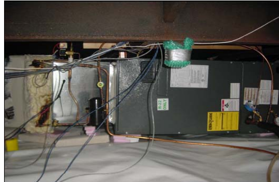
Figure 1- 14 Completed ACDM Indoor unit in the MHLab crawlspace
