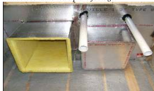
Figure 3- 12 Air barrier in top of air handler closet created with duct board by the mechanical contractor at the time that the ducts are installed.
