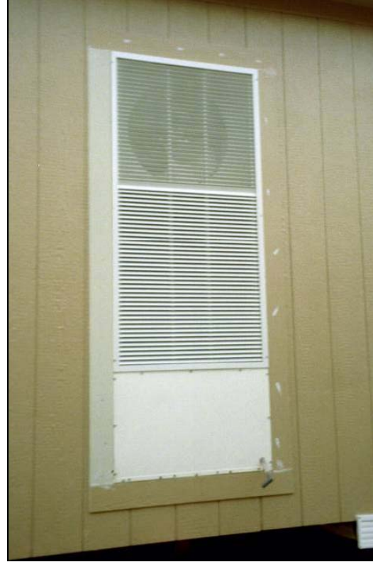
Figure 1- 13 Exterior view of the Comboflair under test in Austin, TX at the Palm Harbor Home model center
