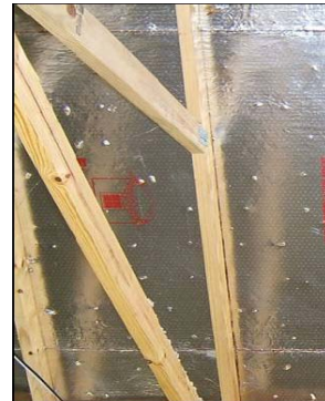
Figure 4- 9 Radiant barrier reduces heat transfer from the roof, a major component of the cooling load.
