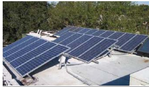
Figure 2- 40 2.25kWp Photovoltaic power system on roof top of 2007 TNAH
