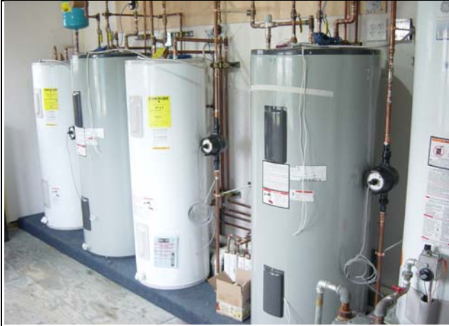
Figure 1- 29 One half of the tanks inside the test shed.
