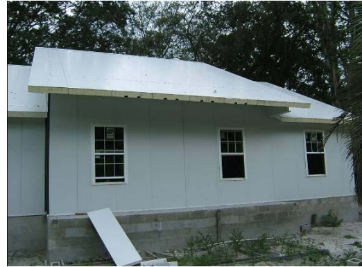
Figure 2-10 Channels in roof construction to allow ventilation of potential heat generated from PV
