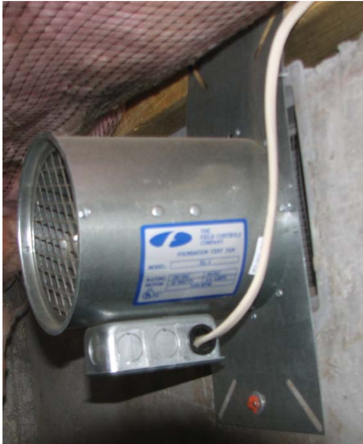
Figure 10 –Crawlspace Fan - Fort Lewis Army Base, Washington
