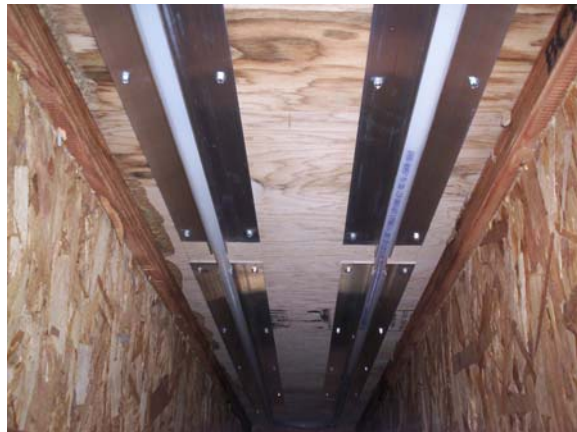
Figure 7a & 7b – Stamets Residence, Radiant Floor Zonal Heating System
