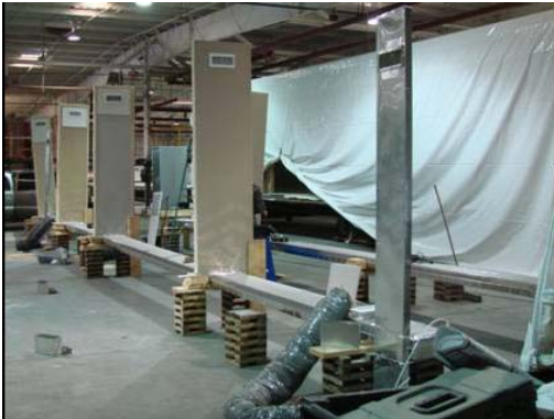
Figure I-3 Floor duct system with high sidedischarge outlets under construction being tested with duct tester
