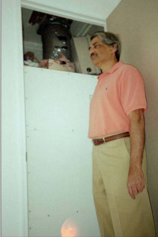
Figure 1- 12 Interior view of the Comboflair System with Mr. Henry Delima, Comboflair project director
