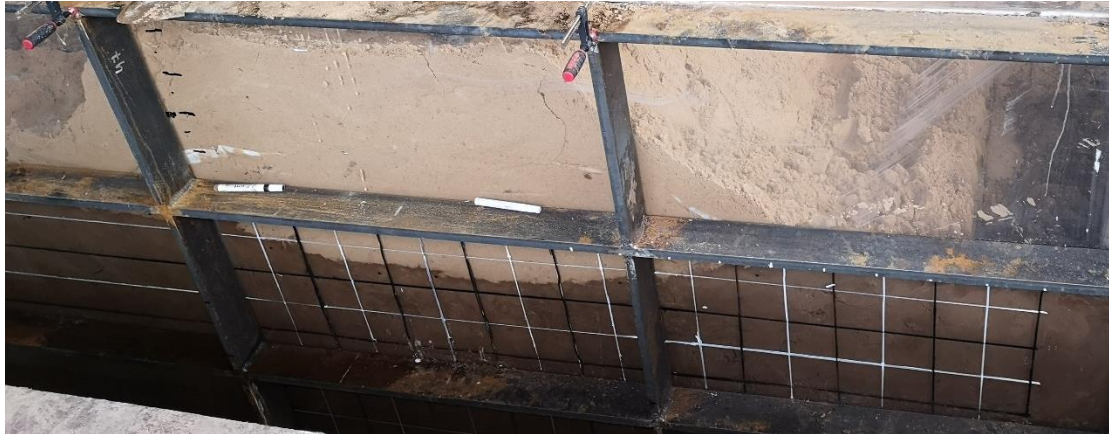
Figure 9. General perspective on the distortion of the base under the scaffold in the wake of testing
