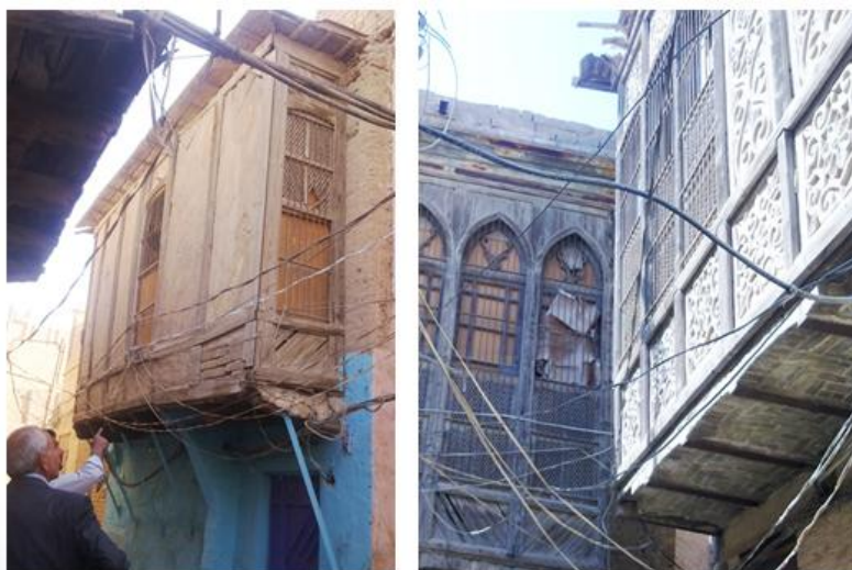
Figure 8. shows the wooden tiered plinth over the arched walls on the ground floor (photographs by researchers)
