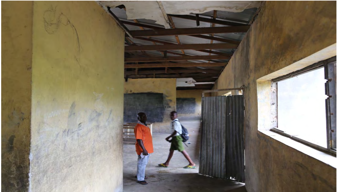
Figure 6. 5 A Dilapidated school in Rivers State
