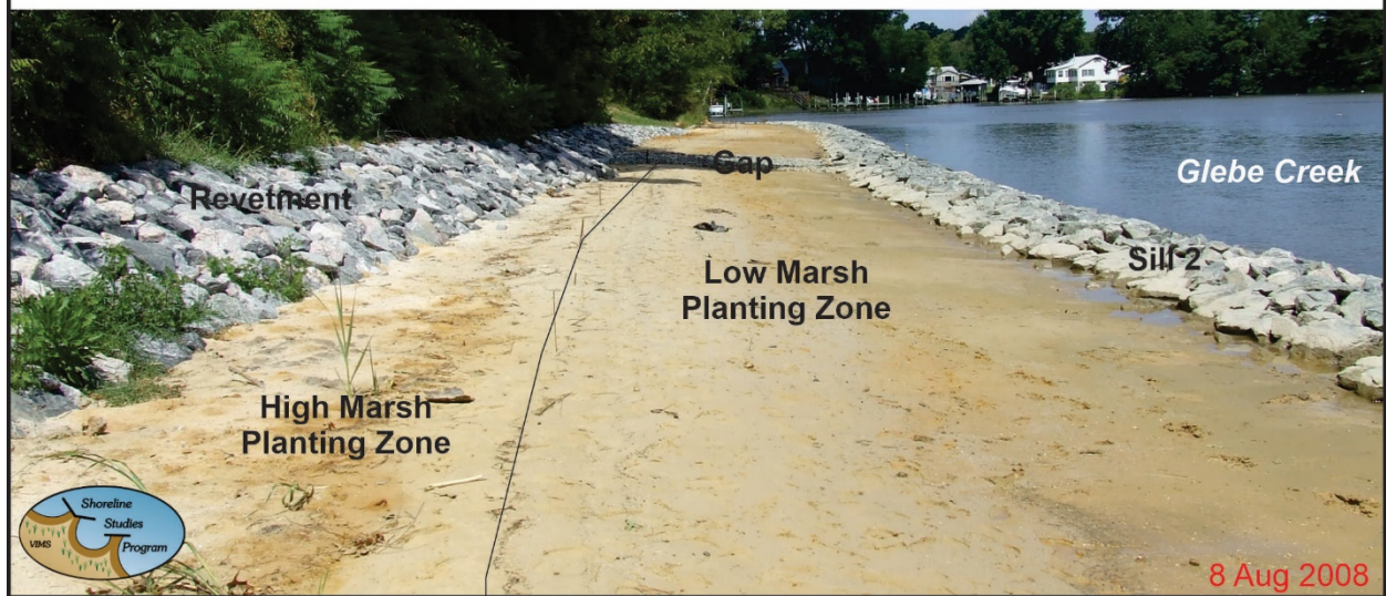
Figure 9-10. Post construction ground photos showing the low and high marsh planting zones. The marsh was planted soon after.
