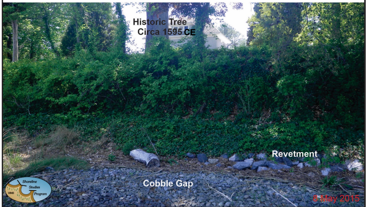
Figure 9-12. Hull Springs Farm about 6 years after construction. Top: Sill 2 has lush low marsh behind the structure, but the high marsh is not as vegetated. Bottom: The bank has slumped over the revetment. The sediment is vegetated which adds additional stability to the bank to protect the historic tree. Photo credit: Shoreline Studies Program, VIMS.
