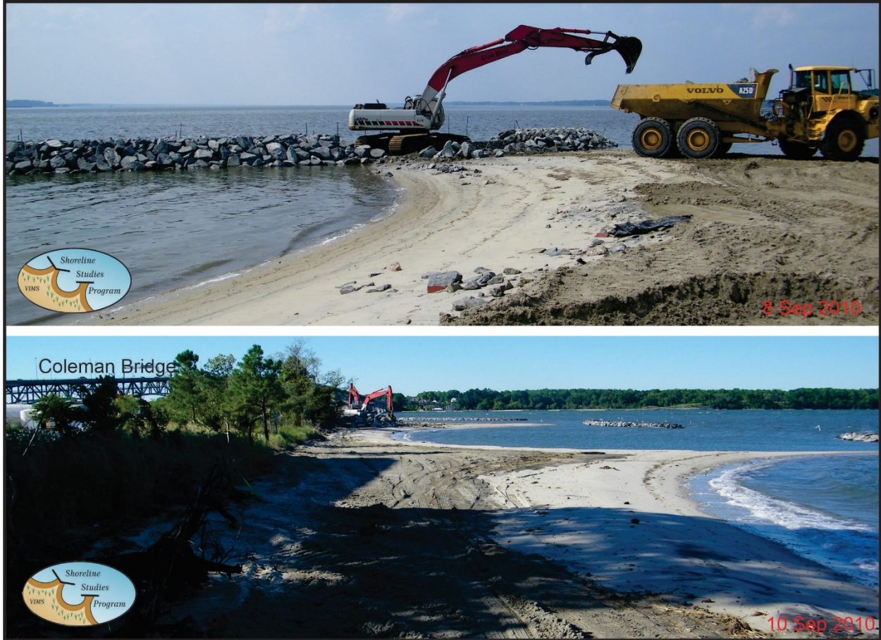
Figure 6-9. VIMS West shoreline during construction of the living shoreline in 2010. Photo credit: Shoreline Studies Program, VIMS.
