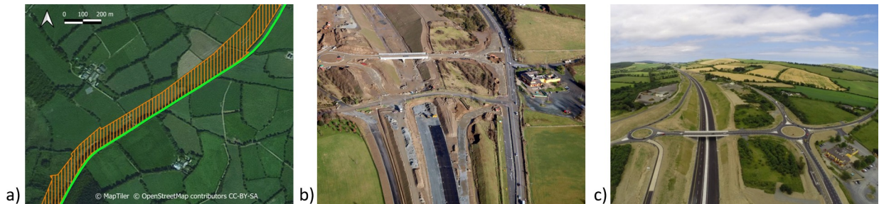
Fig 1. Road construction phases. a) 'Before'—satellite image of part of the study area before road construction. The hatched orange area indicates the location of the M11 motorway construction zone adjacent to the N11 road. The N11 is represented by the green line. b) 'During'—aerial photograph of part of the study area taken during road construction revealing the extent of the change to the habitat. The N11 can be seen to the right-hand side of the photograph. c) 'After'—aerial photograph of part of the study area taken upon completion of road construction. The motorway and access roads were completely enclosed in continuous badger-proof fencing.
