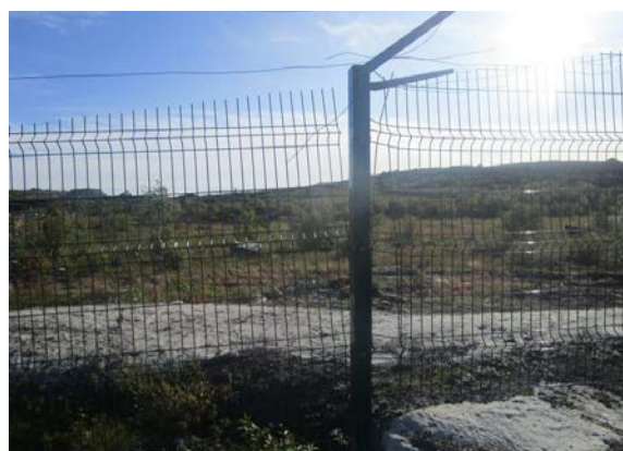
Fig. 2. Destruction of the panel near to the support.
