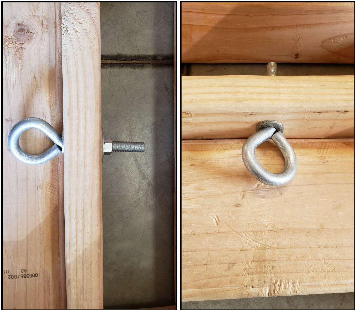
Figure 20: The platform's eye bolt that the winch attaches to
