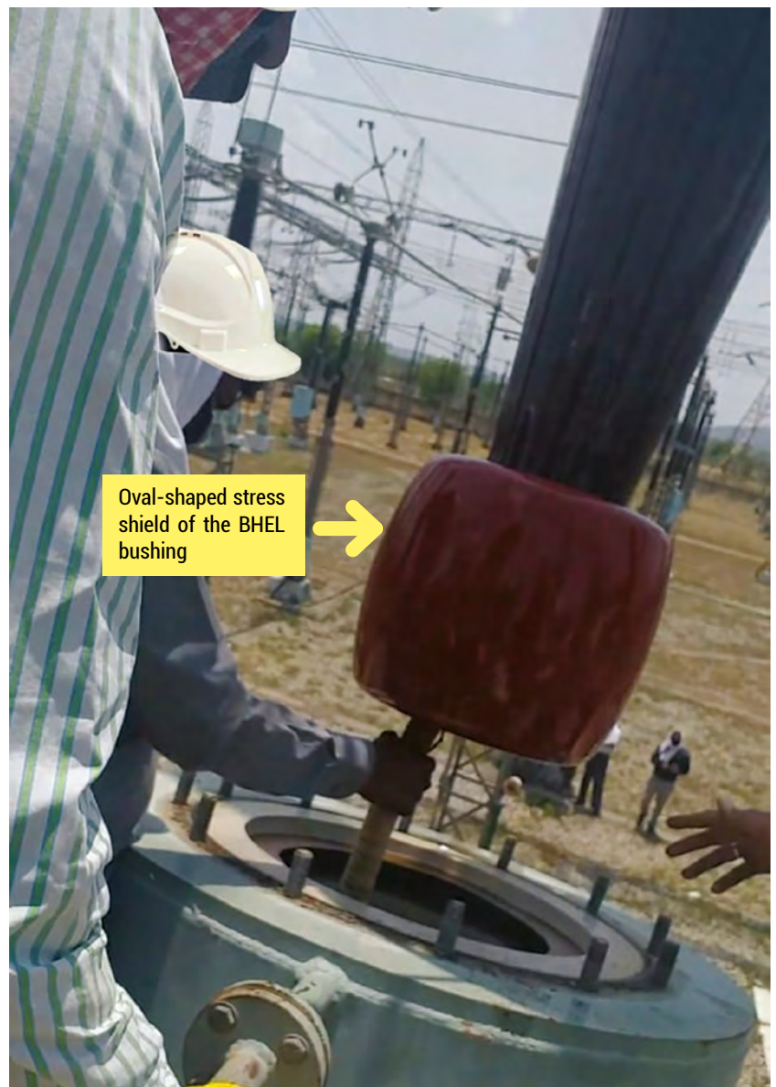
Figure 1. The process of removing the 420 kV BHEL bushing with the Hydra crane.
