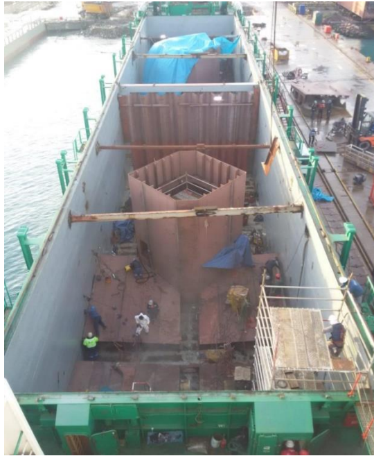
Figure 2 Ship no.1 cargo area photo taken in the shipyard during major conversion and new parts installation into existing hull
