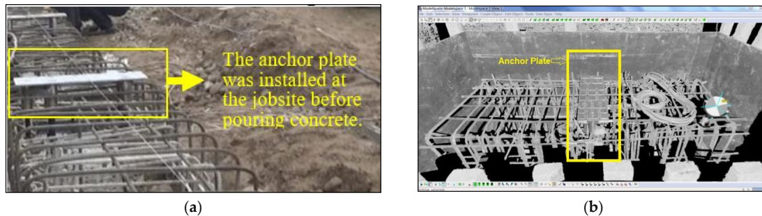
Figure 13. Anchor plate in the job site and point cloud. (a) Anchor plate in the job site and (b) anchor plate point cloud.
