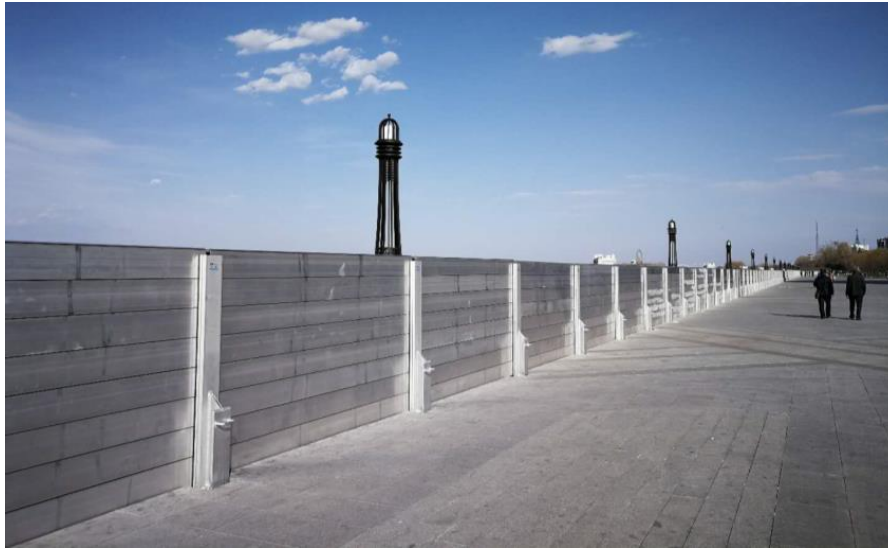
Figure 19. The view of the removable floodwall.
