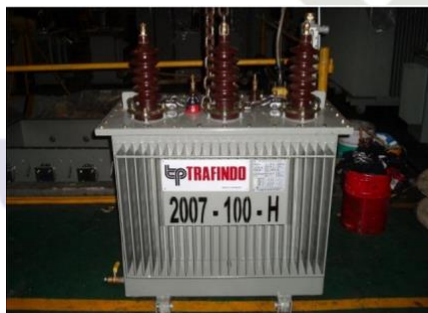
Gambar 2. 21 Transformator Distribusi Off Load Tap Changer [26].
