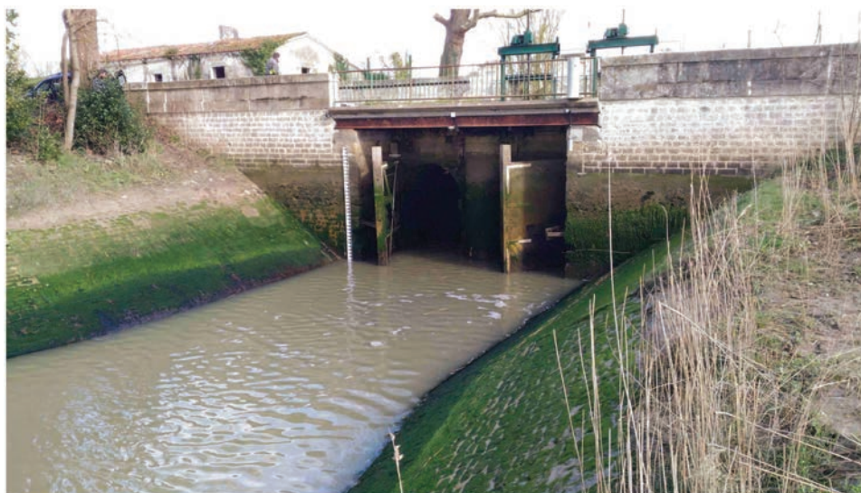
Fig. 1. (Color) Example of tidal door at Charras marsh.
