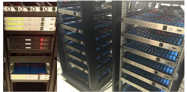
FIGURE 12. (a) Reconfigurable battery pack in UPS replacement in data centers; (b) The first large-scale reconfigurable battery system with 1792 LiFePO4 26650 battery cells.
