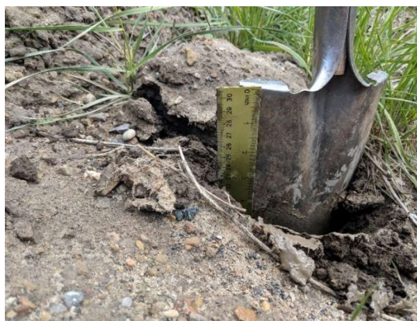
Figure 17. Evaluation of erosion at the bottom of a pock.
