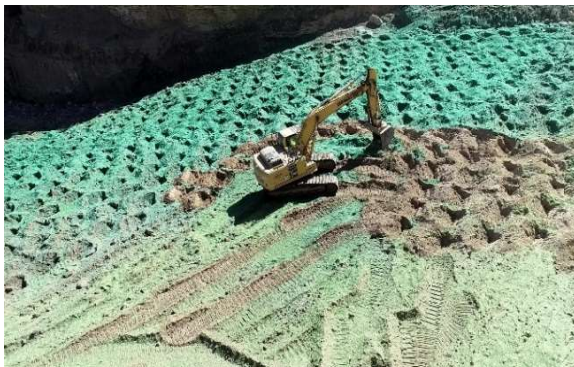
Figure 1. Pocked slope at the Deer Creek Coal Mine reclamation site, Emery.
