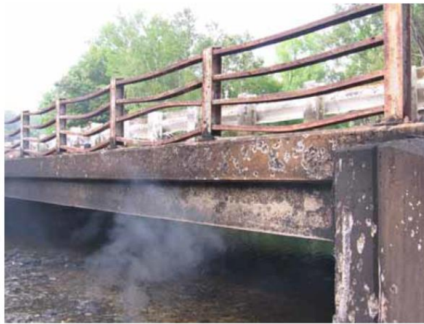
Figure 3.6: Fascia of the bridge after the fire (reprinted from [48])
