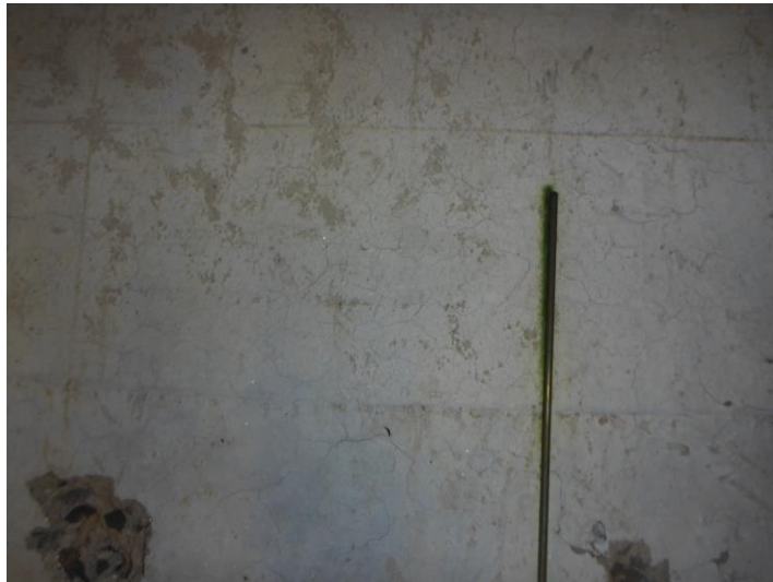
Figure 7.20: Typical map cracking pattern for slabs after heating up to 930°C
