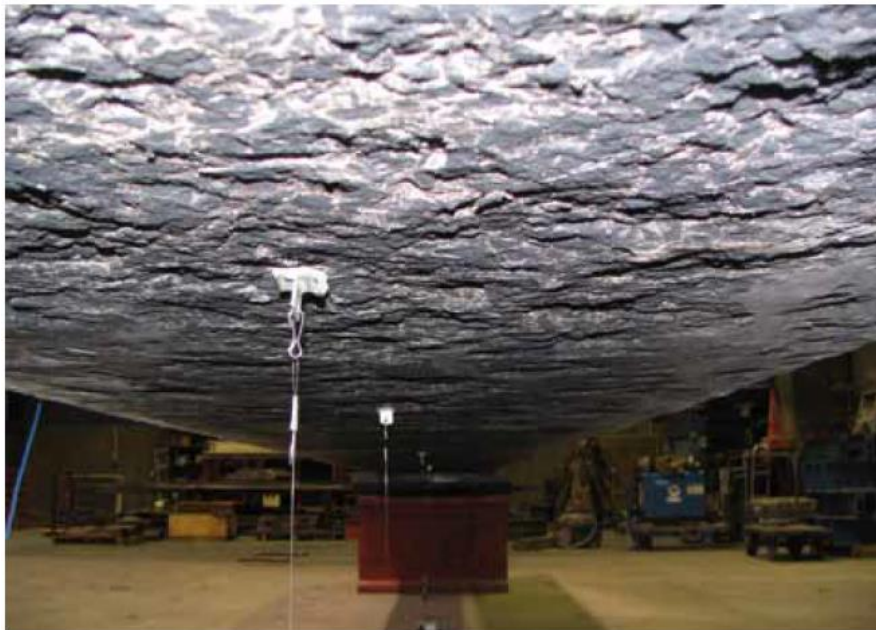
Figure 3.8: Visual condition of the bottom of beam 4 (reprinted from [48])
