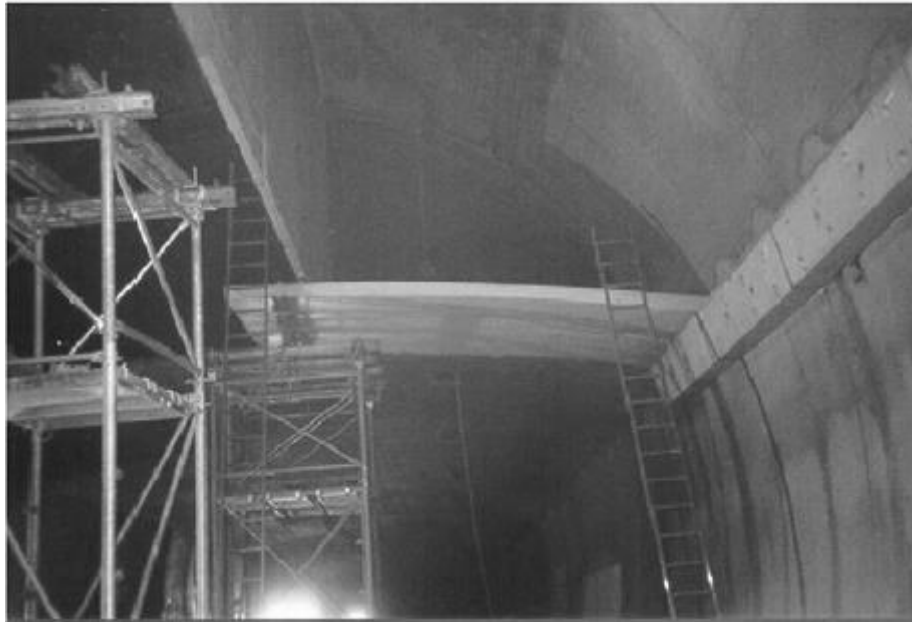
Figure 5.8: Installation of precast ceiling panels (Reprinted from Tunnelling and Underground Space Technology, Vol. 16, No. 3, The fire catastrophe in the Tauern Tunnel: experience and conclusions for the Austrian guidelines, 2001, with permission from Elsevier [90])
