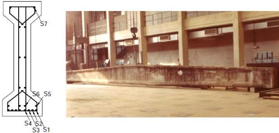
Figure 5.10: Cross-section of pretensioned roof girder (left), pretensioned roof girder after the fire test (right) (Reproduced from fib Bulletin 46, page 129 - “Pretensioned roof girder – cross section and view after fire test,” with permission from the International Federation for Structural Concrete (fib) [8])
