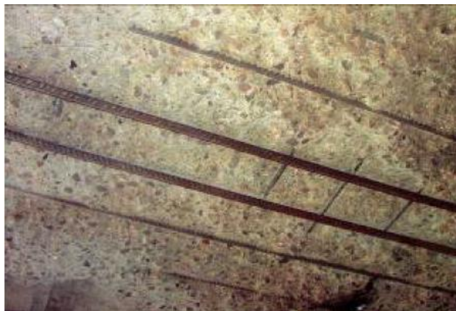
Figure 5.1: Buckled reinforcing bars in the underside of a slab [used with permission from The Concrete Society] [65]
