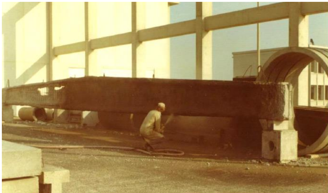
Figure 5.11: Application of shotcrete to damaged girder (Reproduced from fib Bulletin 46, page 130 - “shotcreting of the damaged girder” by Taerwe et al. 2006, with permission from the International Federation for Structural Concrete (fib) [8])
