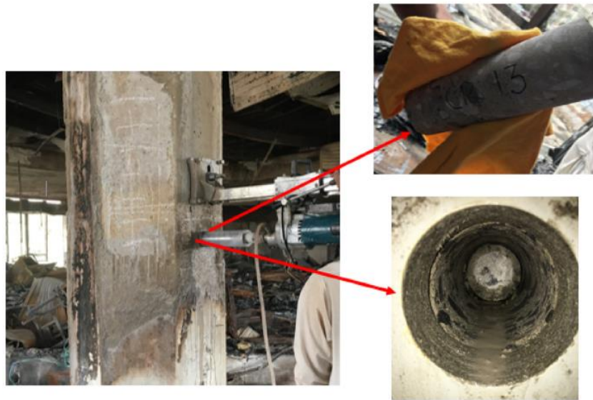
Figure 4.10: Extraction of concrete cores for compressive strength tests (Reprinted from Case Studies in Construction Materials, Vol. 11, Structural health assessment of fire damaged building using non-destructive testing and micro-graphical forensic analysis: A case study, 2019, with permission from Elsevier [75])
