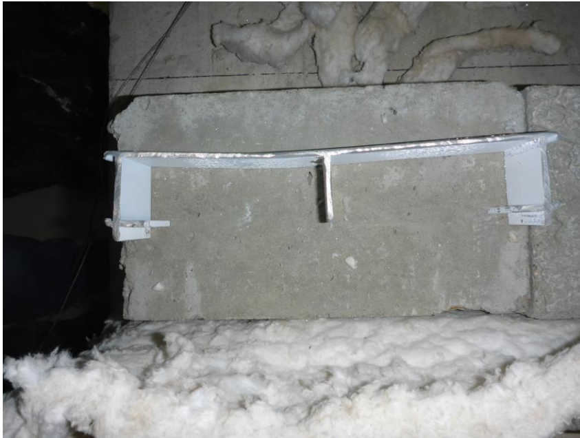
Figure 7.26: Sagging of aluminum wireway after heating
