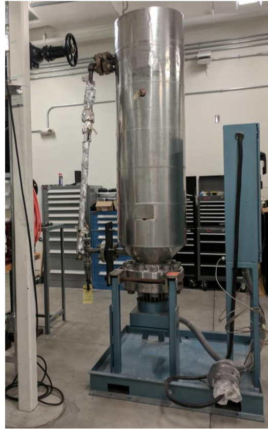
Figure 7. Electric air heater in GDL
