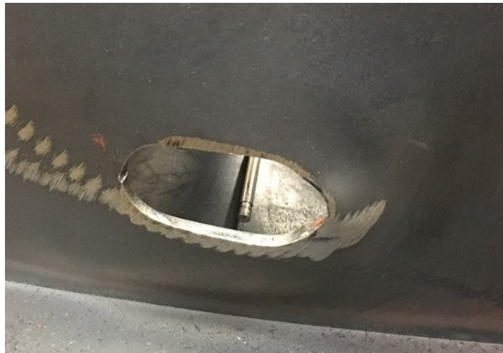
Figure 7-13. Typical web bearing deformation at the hillside washer nipple bearing point (C3 test shown)
