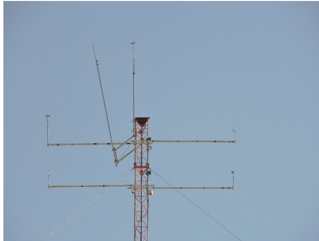
Fig. 3.2 Top section. Top mounted anemometer Thies Clima on top boom at 130 m. Anemometer Thies Clima on L-shaped boom at 125 m and wind vane Thies Clima mounted on an L-shaped boom at 125 m. Anemometer Young on L-shaped boom at 122 m and wind vane Thies Clima mounted on an L-shaped boom at 122.
