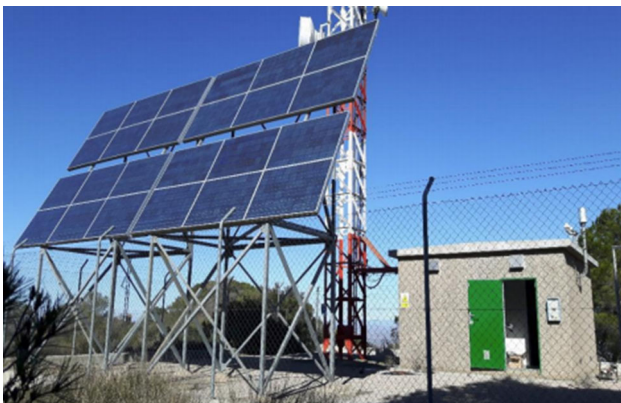
Fig. 1 PV installation in Sigena, region of Aragón, Spain
