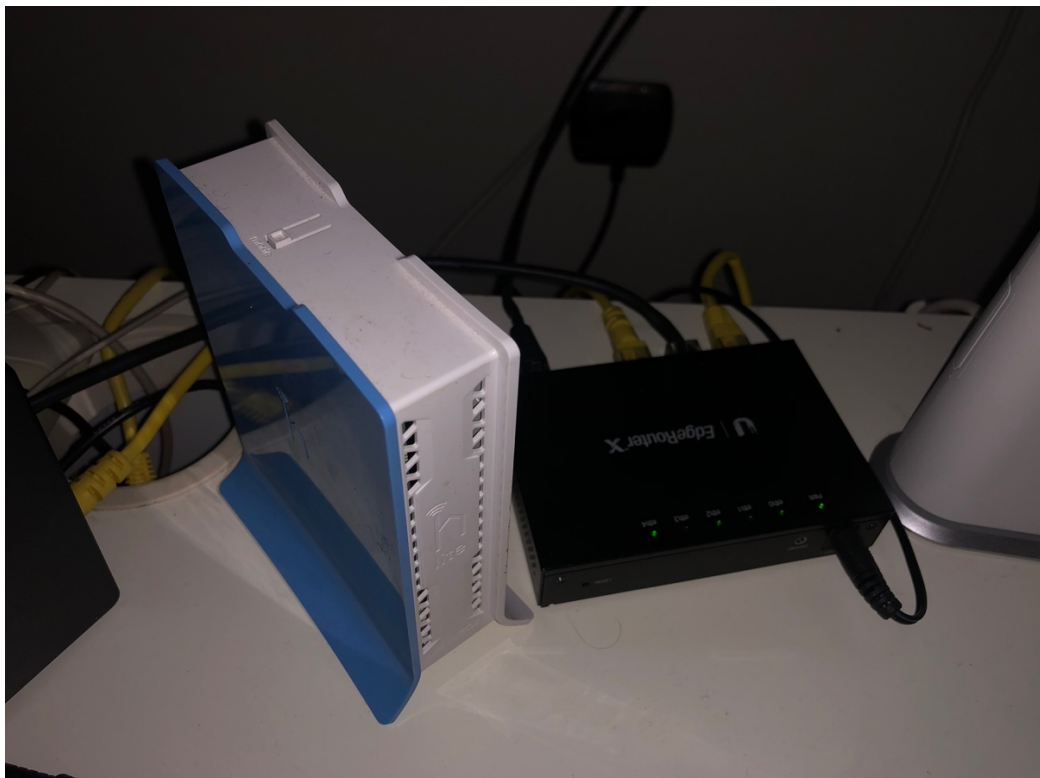
Physical Middleboxes: Edgerouter ER-X and Mikrotik hAP lite
