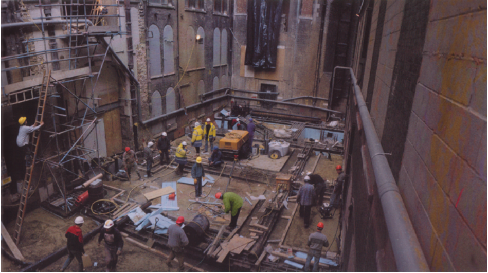
Fig.04. This image is titled 'High View, Construction of the Floor Slab for the Lecture Theatre'
