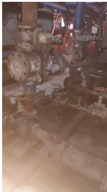
Gambar 2.14 Feed Water Pump
