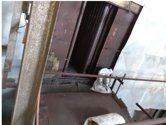
Gambar 2.12 Air Heater Pipe
