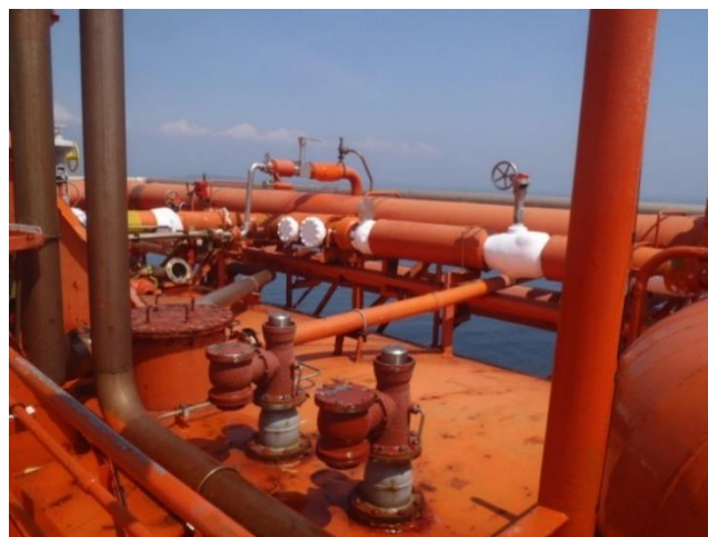
Figure 2.1 Icing in LNG Pipeline (Source: Personal Documentation at FSRU Jawa Barat, Nusantara Regas)
