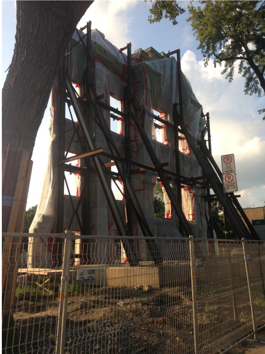
Figure 78. The entryway of the École Baril, after the demolition of the surrounding structure in May 2015. Personal photograph.
