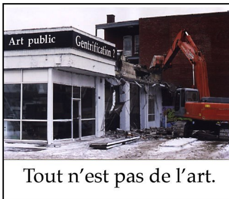
Figure 75. The 2002 demolition of Garage de la culture/Rozon Garage, as represented in Gilles Bissonnet’s mural Tout n’est pas de l’art . In 2003, Bissonnet installed the mural on the site of the former Garage de la culture/Rozon Garage during L’Urbaine Urbanité II . From Tout n’est pas de l’art [Digital photograph with text], by G. Bissonnet, 2003, Private collection of the artist. Copyright 2003 by Gilles Bissonnet. Reprinted with permission.
