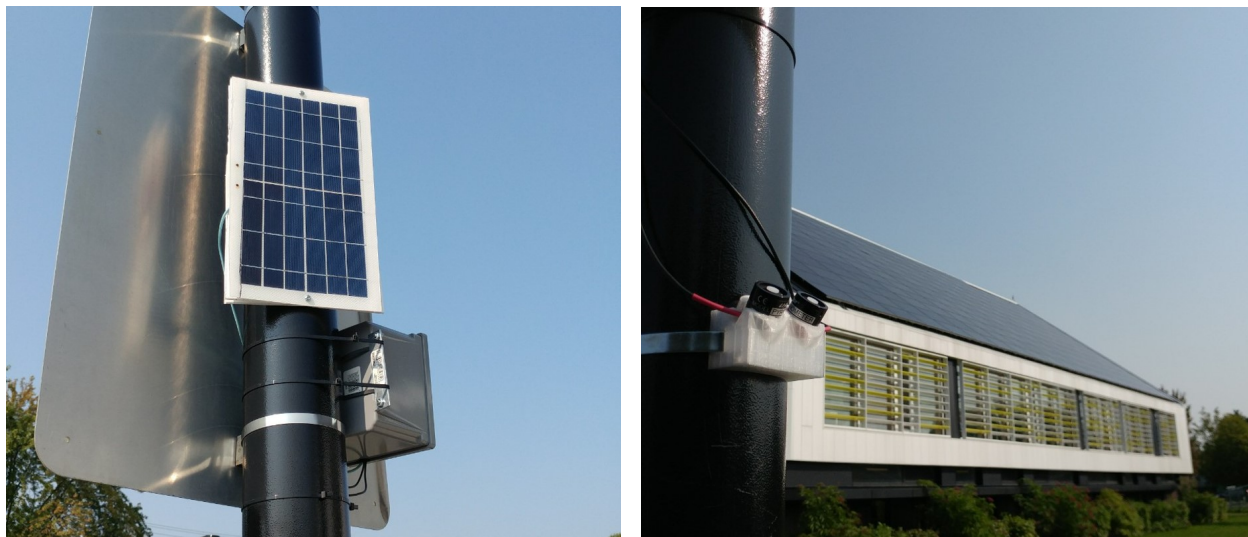
(a) Small PV panel charging control box battery seen on the right of the pole
