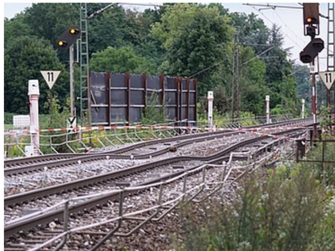
Figure 1.1. Collapsed sinkhole beneath the existing surface rail tracks and buckled railway tracks (Shani and TunnelTalk 2017).
