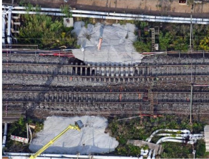
Figure 1.2. Concrete backfills the collapsed tunnel (Shani and TunnelTalk 2017).
