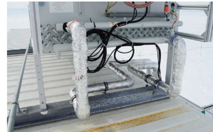
Insulated thermal piping connecting to the free cooler on top of the MTF
