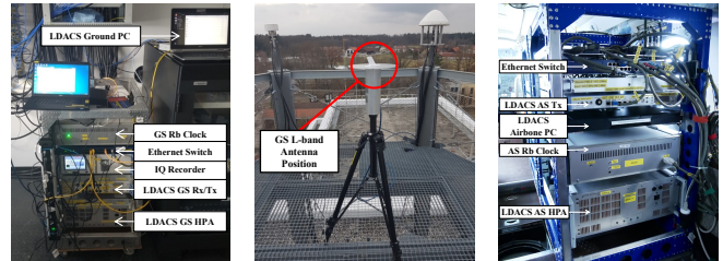
(b) Ground station (c) LDACS antenna (d) A/C installation
