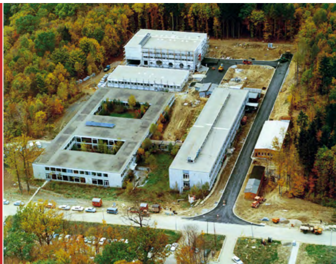
And the excavators keep on rolling – the buildings for the Institute for Plasma Dynamics and the central workshop were built in 1967.
