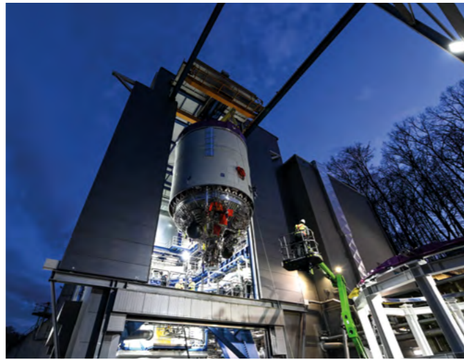
The upper stage of the Ariane 6 launcher is integrated into the new P5.2 test stand at DLR's Lampoldshausen site.
