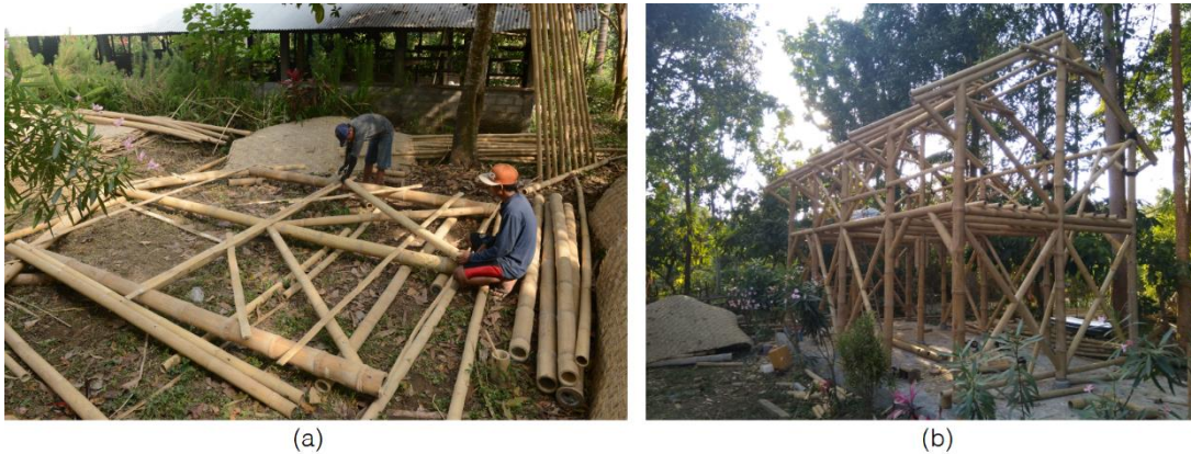
Figure 2.12. Bamboo pole structural frame being assembled on the floor (a), followed by the subsequent structural skeleton of a house (b)
