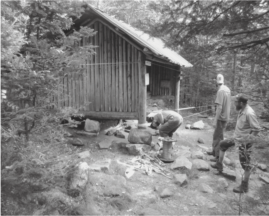
Joe Roman (left), Declan Scannell, and James Vittetau rig up the Ethan Pond Shelter with an iron rope in preparation for hoisting it back into plumb. SALLY MANIKIAN
