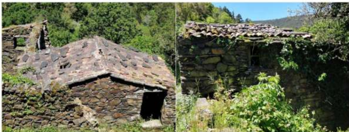
Fig. 3. SE and NE views of the ancient dwelling to be restored (S. Carneiro)
