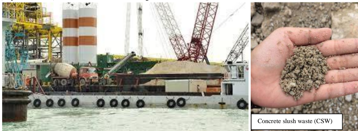
Fig. 3 - Durable Mix Concrete Batching Plant, Panchor, Muar, Johor
