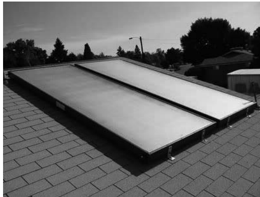
Figure 6-3. A Typical Roof-Top Solar Collector (courtesy of U.S. Dept. of Energy)
