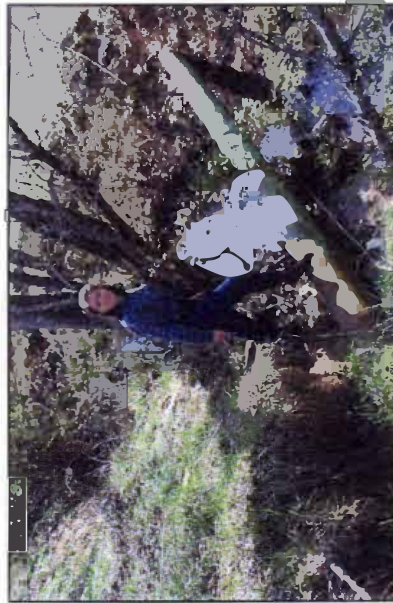
B. An exposed sewer line at TS01.
