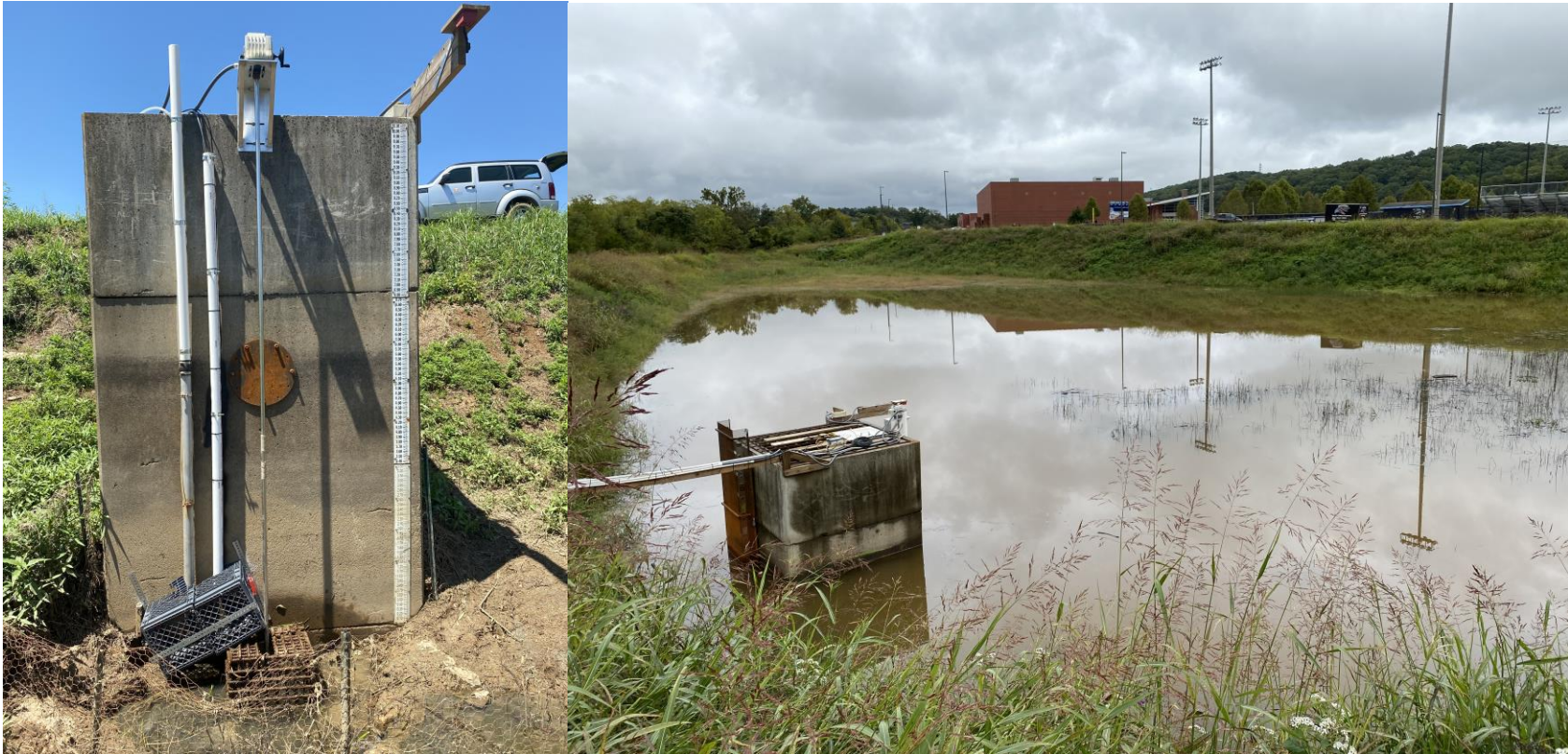
Figure 3.2. Dry extended detention basin outlet riser (left) outfitted with controllable valve, water depth sensor, and turbidity sensor and (right) the basin following a rainfall event.
