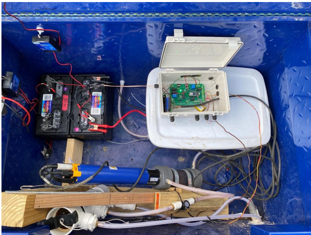
Figure 4.2. Top-down view of water quality instrumentation including EXO2 in flow cell (bottom center), custom control circuit for wirelessly uploading data (top right), peristaltic pump (top right - inside white tub), and deep-cycle batteries for power (top left).
