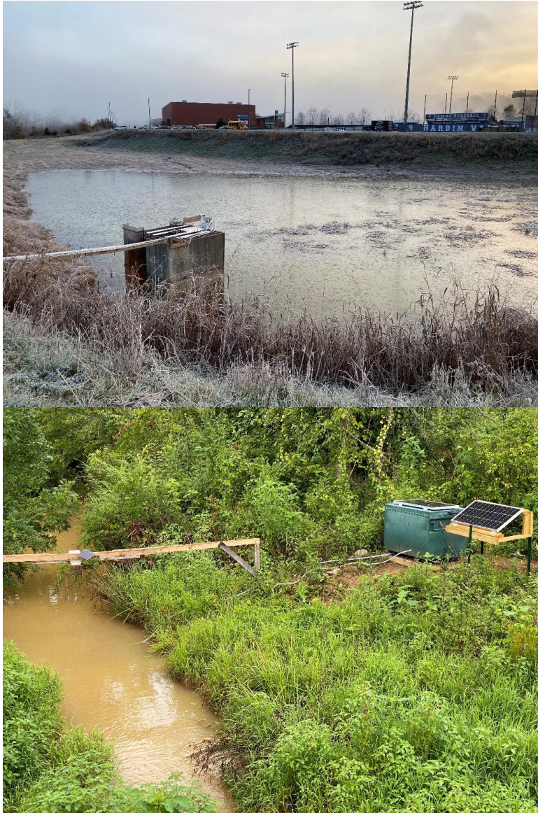
Figure 4.1. Dry extended detention basin (top) retrofitted with a controllable valve, water depth sensor, and rain gauge following a rainfall event and (bottom) the downstream monitoring location outfitted with a custom stream gauging station and water quality instrumentation.
