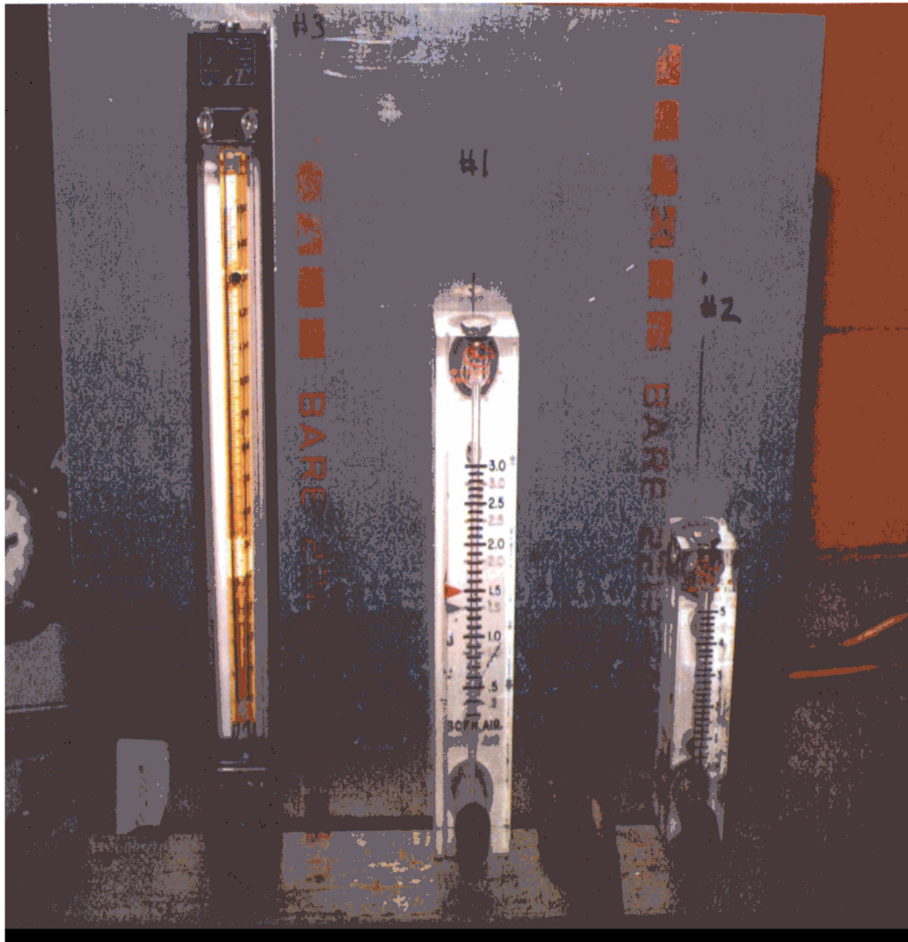
Figure 11. Flowmeter Panel – Flowmeter in each Rivulet Water Supply Line
