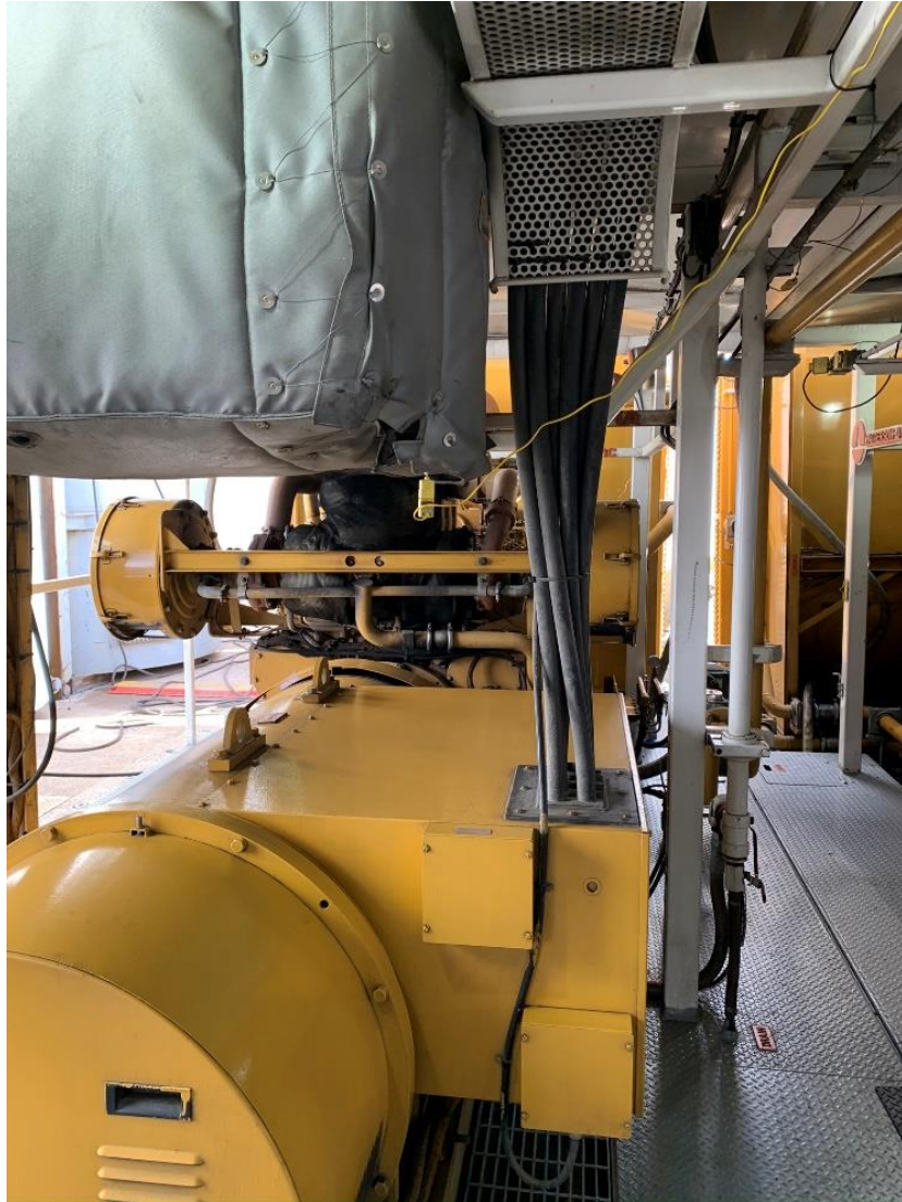
Figure 8. K-Type Thermocouple Installed in the Engine’s Muffler
