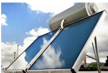
a) ST system for heating water
