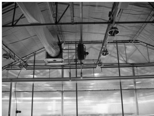
Fig.8. – Unit heaters, (Ponce et al., 2015)
