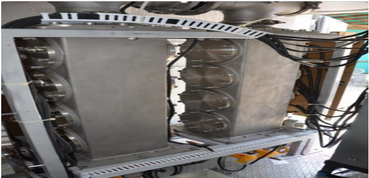
Figure 6.2: 48kW electro-chemical reactor with dual power supplies
